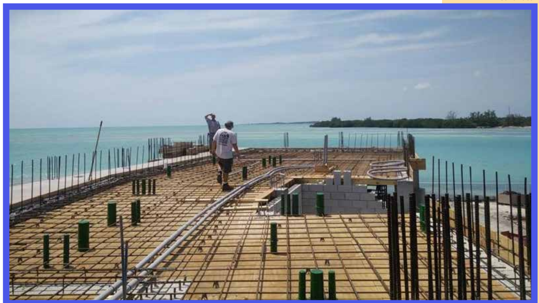
The team lays PVC pipe for elevator power cables during a site visit.
